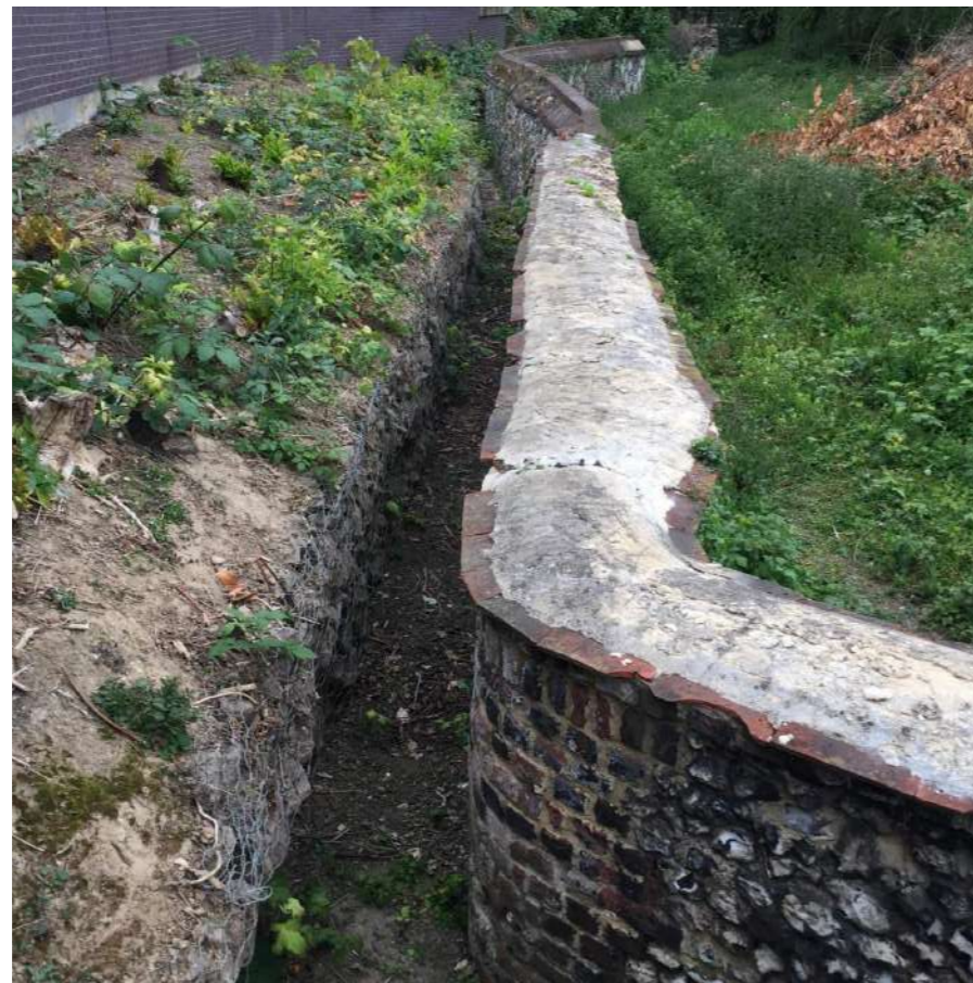
Existing condition - Insufficient / Failing gabion wall
